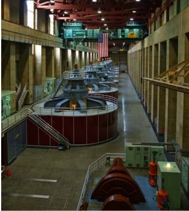
Electric Power Generation
