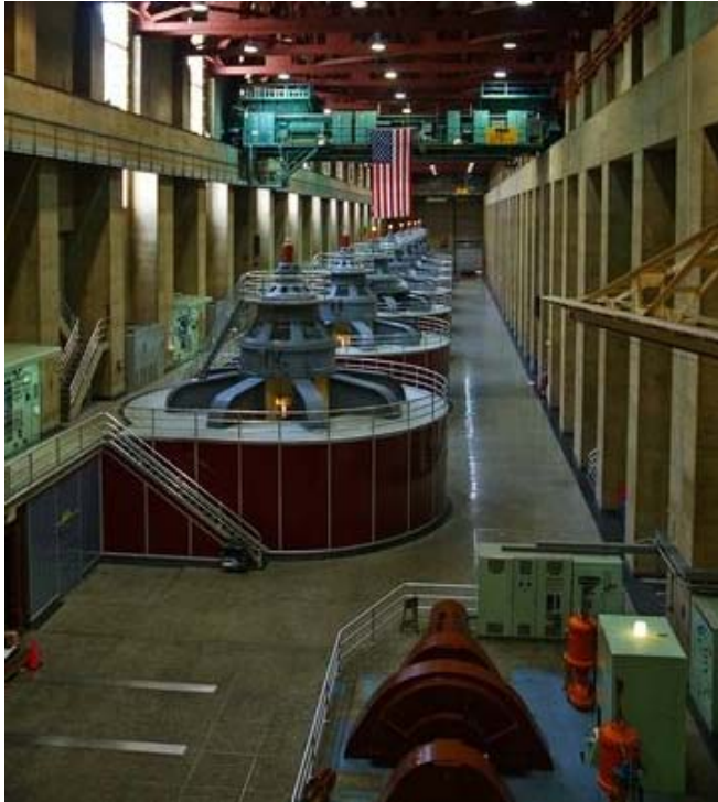
Electric Power Generation
