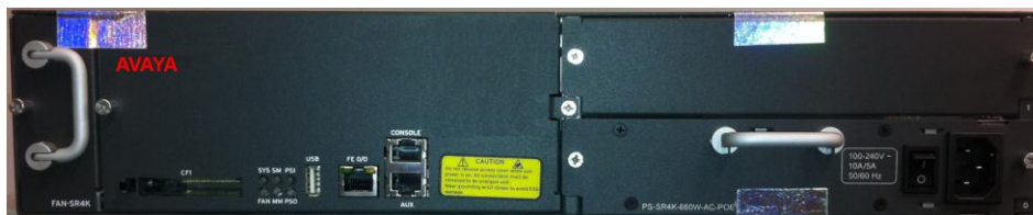
Figure 5 – Rear-end Tamper Evident Labels-1, 2, 3
